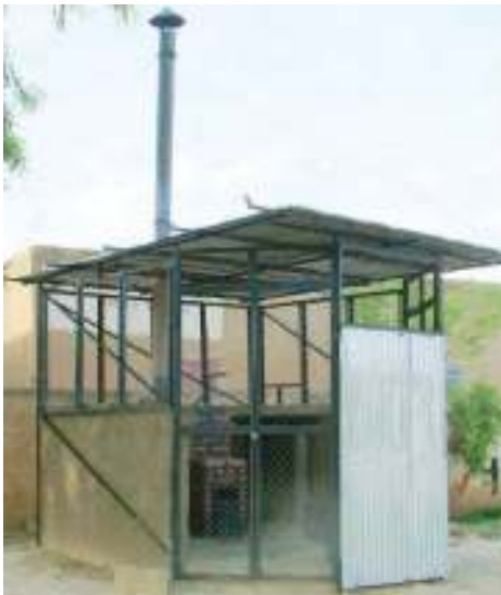
Incenerator ruang ganda
